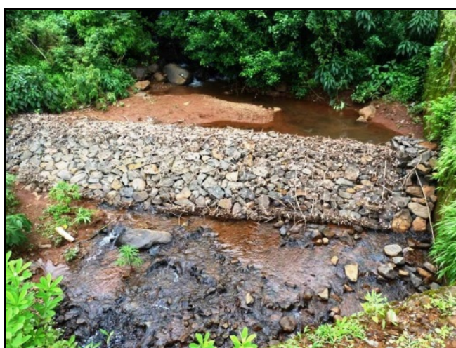
Figure 10.2 d : Illustrative Gabion Structure in Operation
