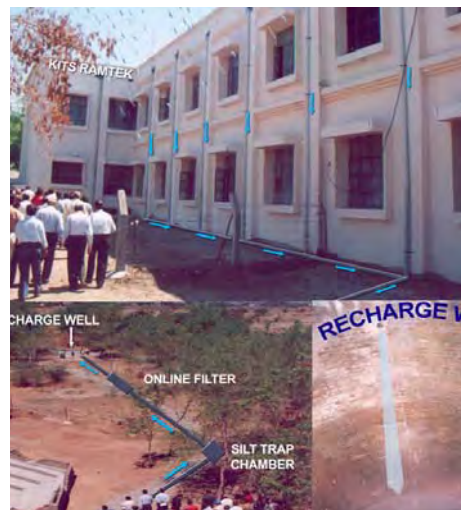
Figure.36. AR structures shaft with recharge well.
