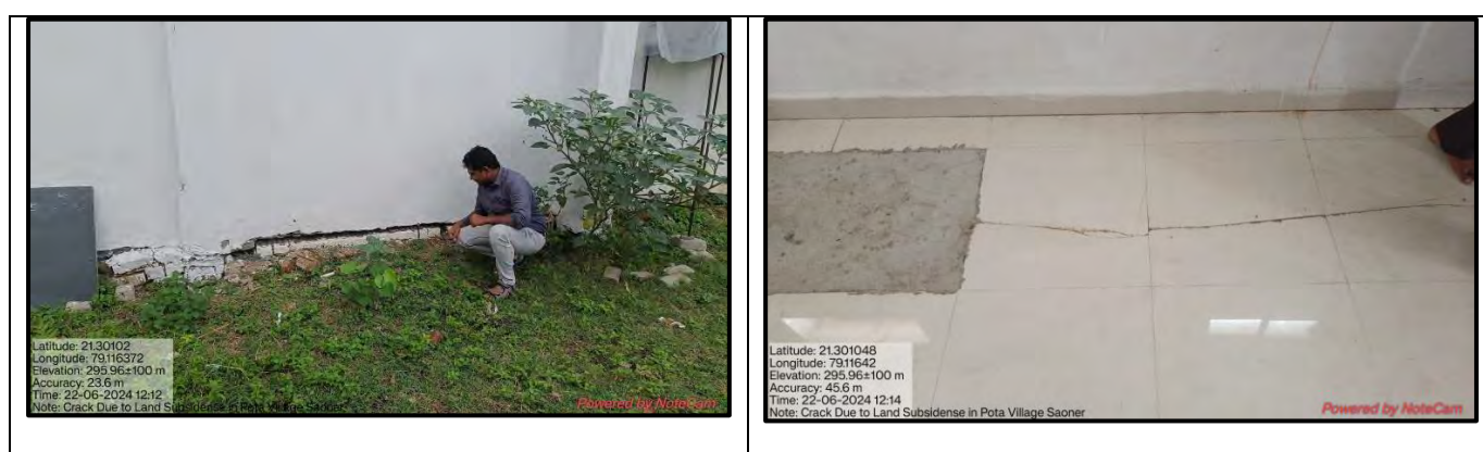
Fig. 9.5 Cracks in foundation and pavements due to land subsidence in Pota village, Saoner
