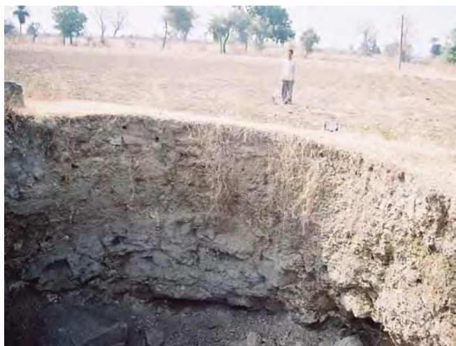
Collapsed well in farmers field at Chikmoh
