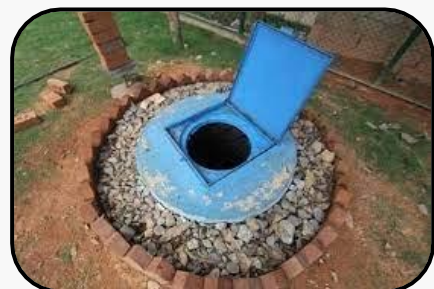
Use of drums in recharge pits
