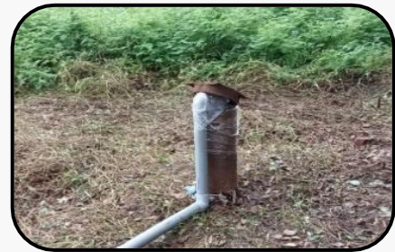
Use of unused borewells for groundwater recharge
