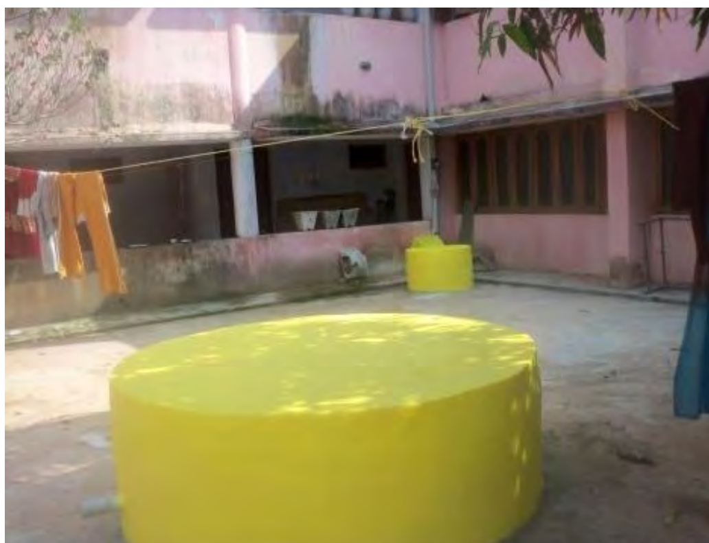
Filter Cum Collection Chamber
