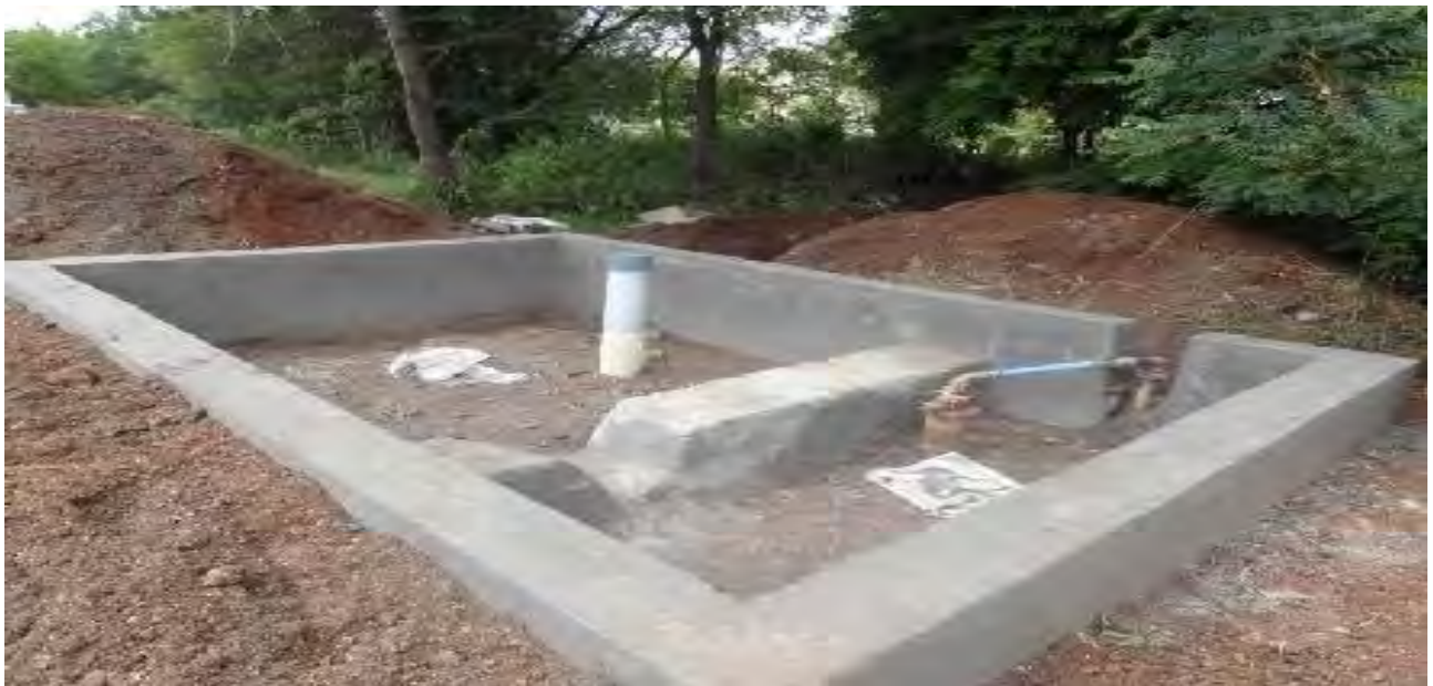
Recharge Pit with Existing Bore Well
