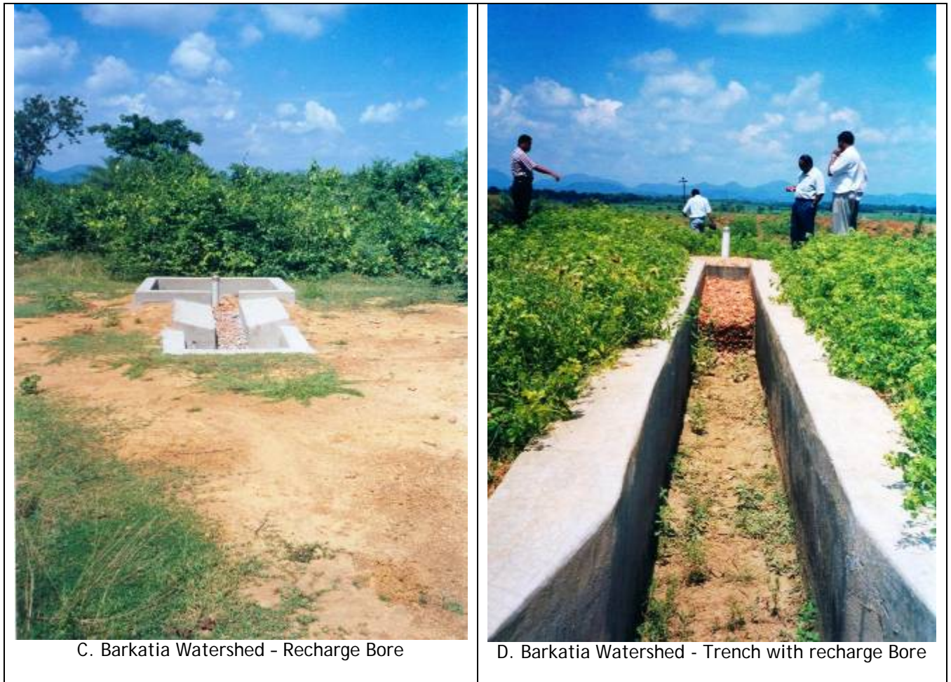
Figure 4.5 (A-D): Artificial Recharge Structures, Barkatia Watershed, Athgarh Block, Cuttack District
