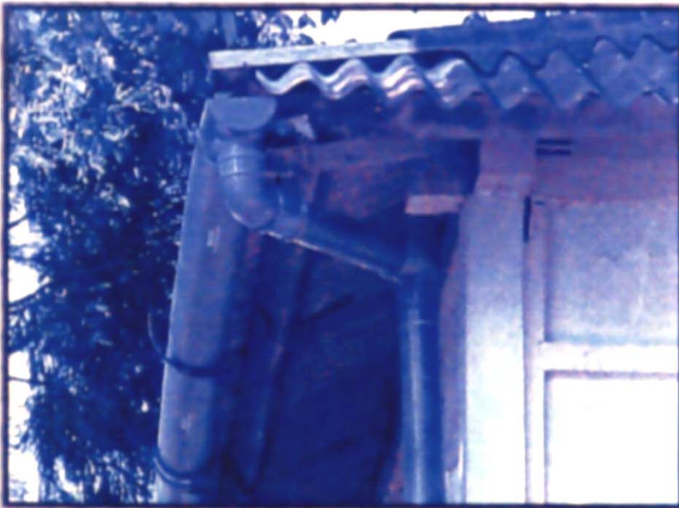
ROOF TOP RAIN WATER COLLECTION POINT
